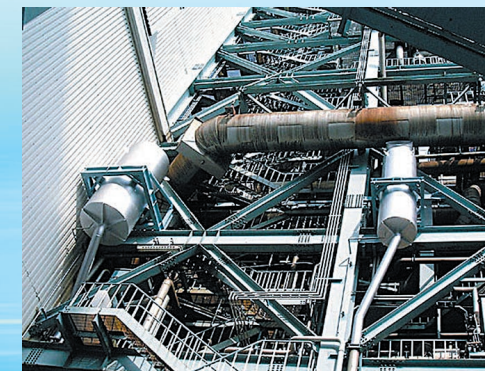
▲ボイラ蒸気安全弁サイレンサ Boiler steam safety valve silencers
